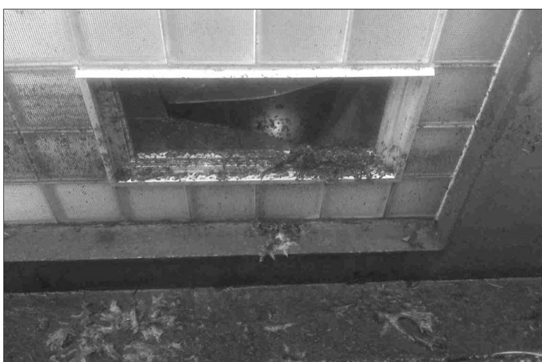
Rain water broke a window on the northeast side of Pershing Building during Midterm Break, causing the lower level multipurpose room and the training room to flood. Photo submitted
