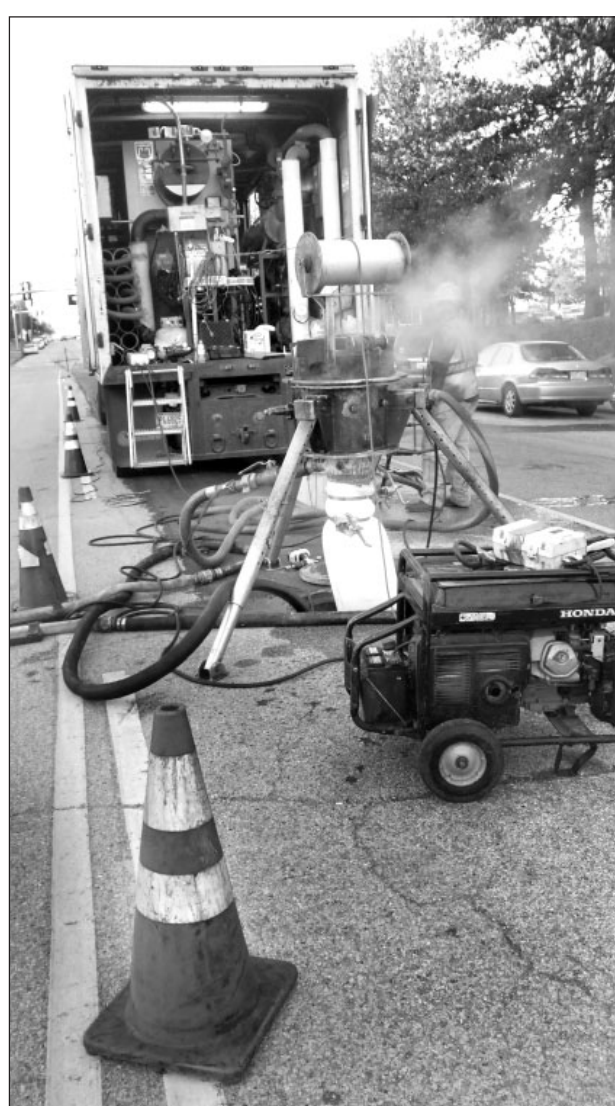
Mayank Dhungana/Index Construction crews work on sewer lines along Franklin St. Wednesday evening. Crews are re-aligning the sewer lines.
