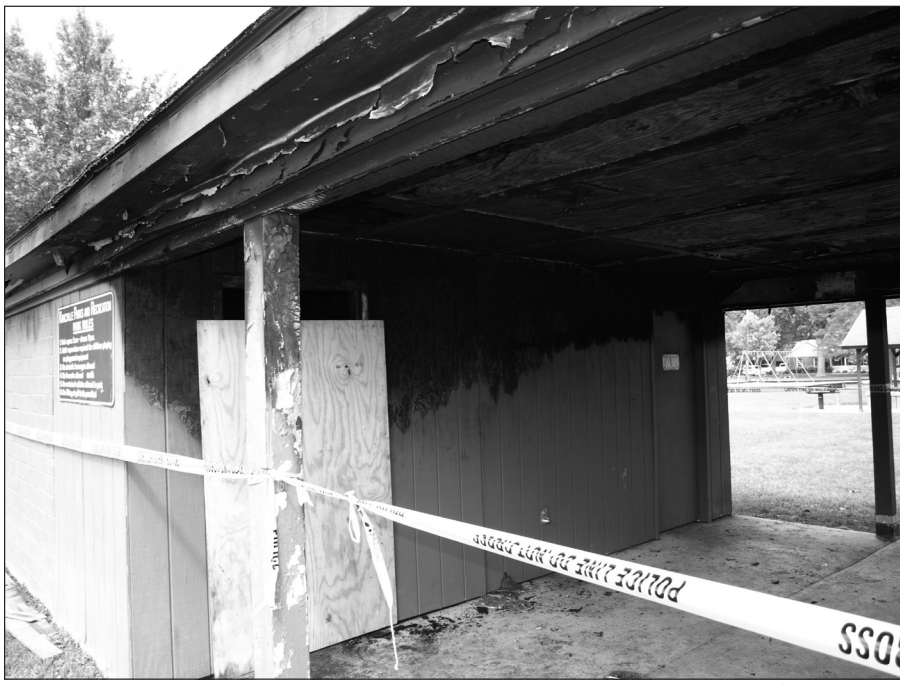
The fire destroyed about 50 percent of the restroom facility. Portable restroom facilities will be available through the end of October.
