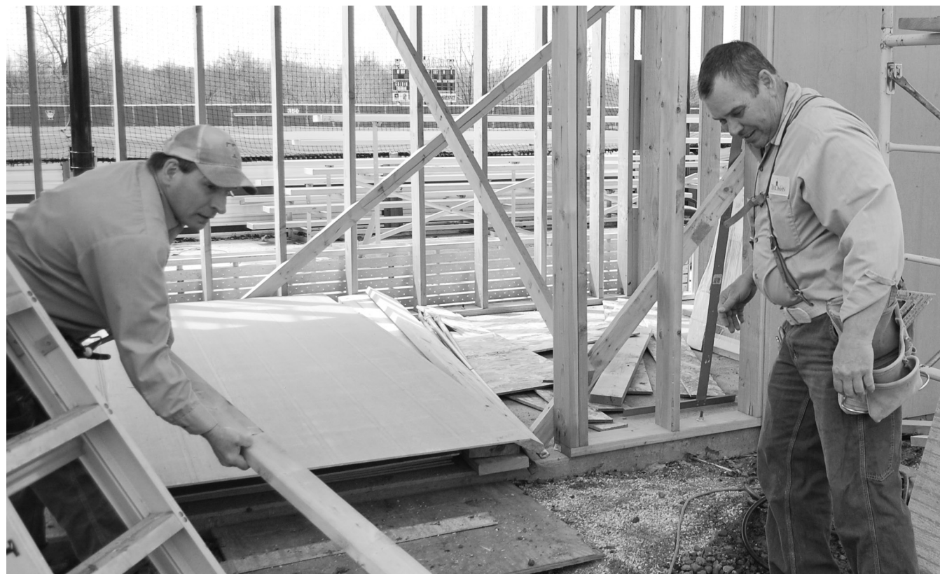
Physical Plant workers Kelly Elsea, left, and Marty Jacques, right, work Monday April 7 on the new press box at Bulldog Baseball Field. The new press box should be completed within the next few weeks, weather permitting. Calie Holden/Index
